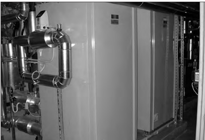
A solar driven absorption cooling system is used at the German Traffic Ministry in Berlin, Germany. Pictured are the absorption machines (2 x 35 kW cool ) and the flat plate solar collectors (229 m 2 ).
