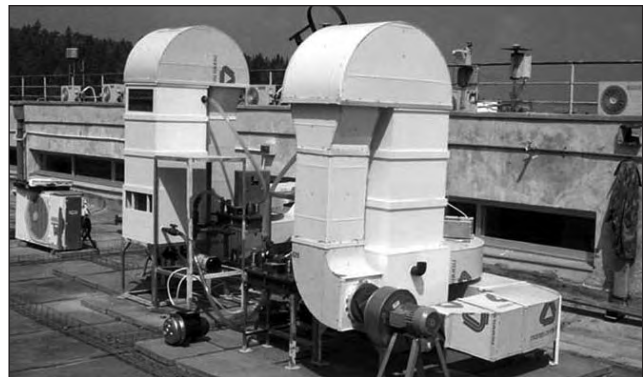
The pilot system using liquid desiccant technology at Technion in Haifa, Israel. Pictured are the liquid desiccant system (4,5 kWcool) and the solar flat plate collectors (20 m 2 ).
