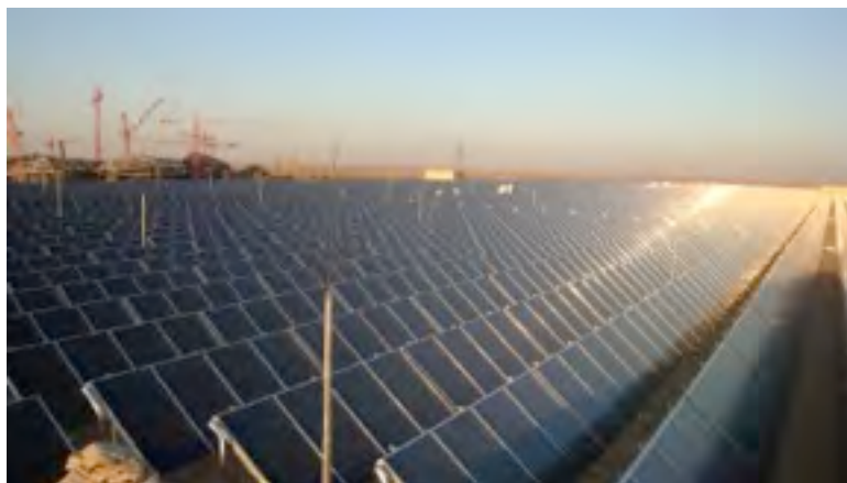
25 MW solar thermal plant at the Princess Noura bint Abdul Rahman University in Riyadh, Saudi Arabia
