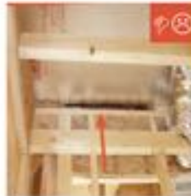
B. Seams of air barrier not sealed.
