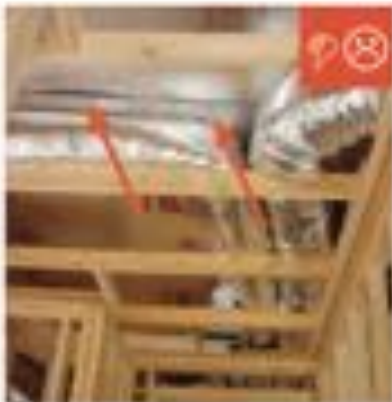
B. Seams of air barrier not sealed.
